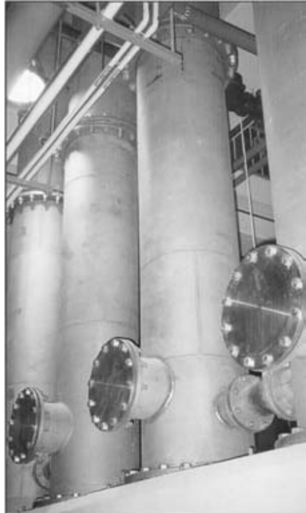
Figure 3 Typical stainless steel chlorine/ozone mixing towers
