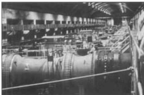
Figure 2 A gallery of laterals in the New York City pumping station. The laterals are made from cast stainless steel with 48 in. diameter wrought butterfly valves.
