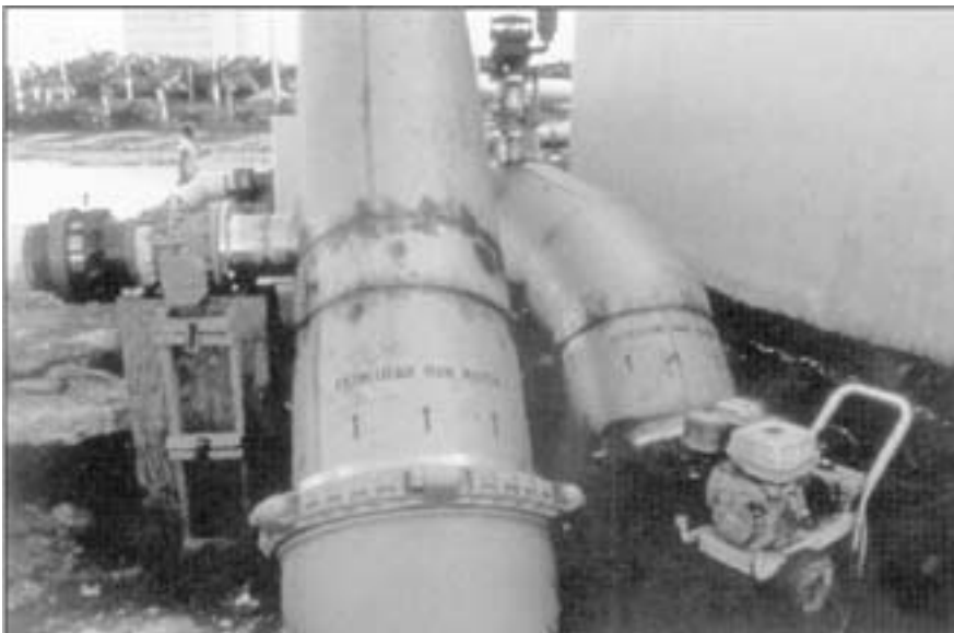
Figure 5 Rust on welds from wire brushing with carbon steel wire brush.
