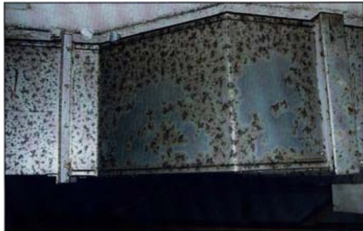
Inspection of the underside of this air ducting revealed corrosion
