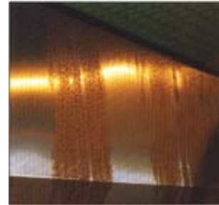
Staining on ventilation trunking
