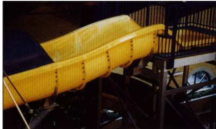
Corrosion attacking the bolts of a flume
