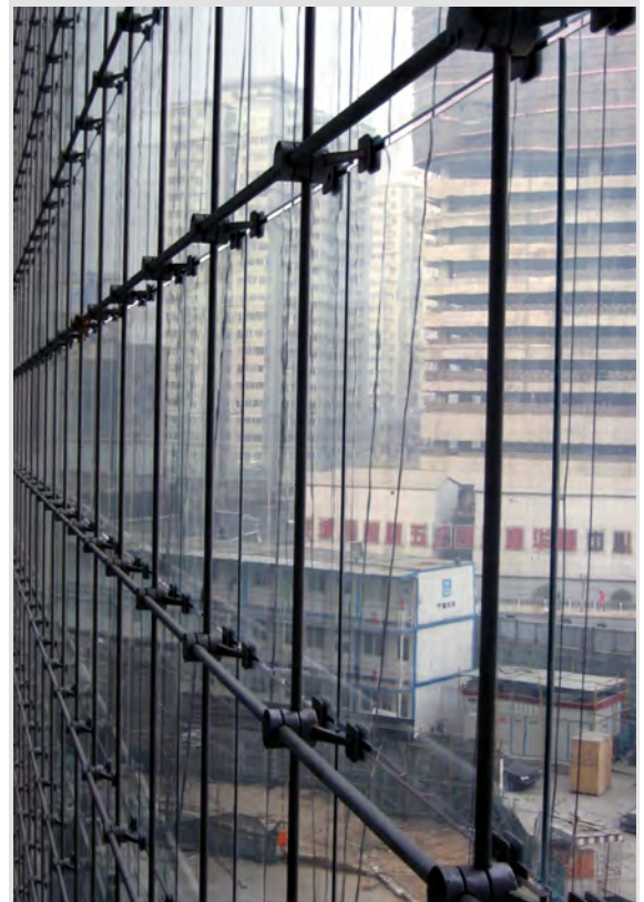
Figure 3: View of the cable-net components including support armature (Photo: Skidmore, Owings & Merrill LLP)
