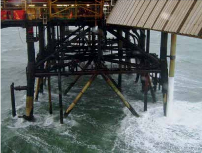
90-10 copper-nickel splash zone protection on a platform in the Morecambe Field, UK. The sheathing has been in service over 25 years (Courtesy Centrica Energy Upstream, East Irish Sea)
