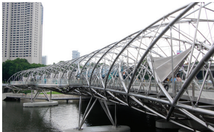
Figure 11 Marina Bay Bridge in Singapore constructed entirely of 2205 duplex stainless steel [Courtesy of Outokumpu Stainless AB]
