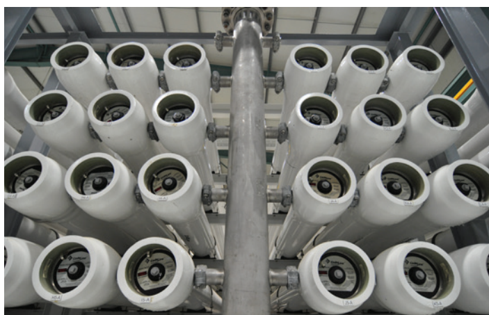
Figure 12 Superduplex piping in a Seawater Reverse Osmosis desalination plant [Photo courtesy of Rolled Alloys]
